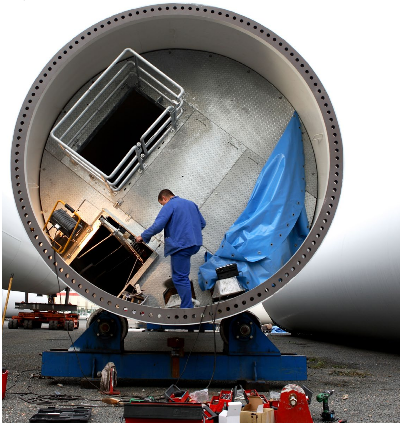
Installation of a lift on a wind turbine on the Harfleur enterprise zone.
