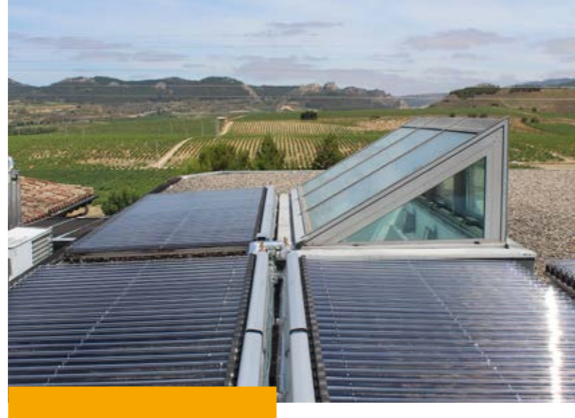
The Spanish solar thermal market is one of a kind in the European Union as it is shared by all solar thermal technologies: conventional flat glazed collectors along with prefabricated thermosiphon systems, vacuum tube collectors, unglazed collectors, as well as hybrid PV-T collectors and solar air collectors.
